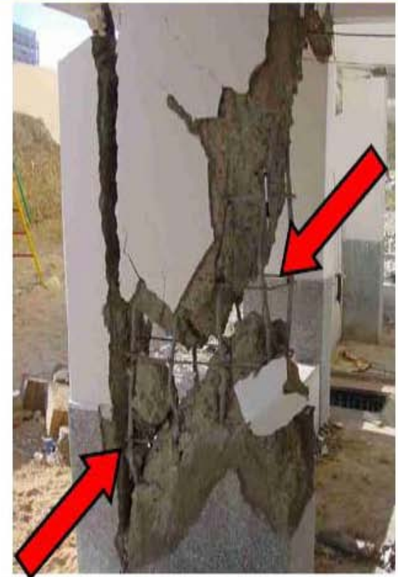
Figure 2: Diagonal cracks in columns jeopardize vertical load carrying capacity of buildings - unacceptable damage.
